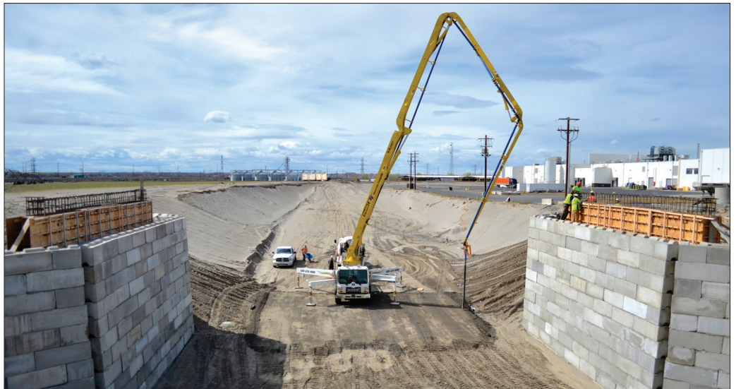
Crews prepare to pour concrete for the stem walls on the Lewis and Clark Drive bridge project. This project is funded by H.B. 2001 – a state transportation bill passed in 2009 – and is planned to be complete by the end of May.
