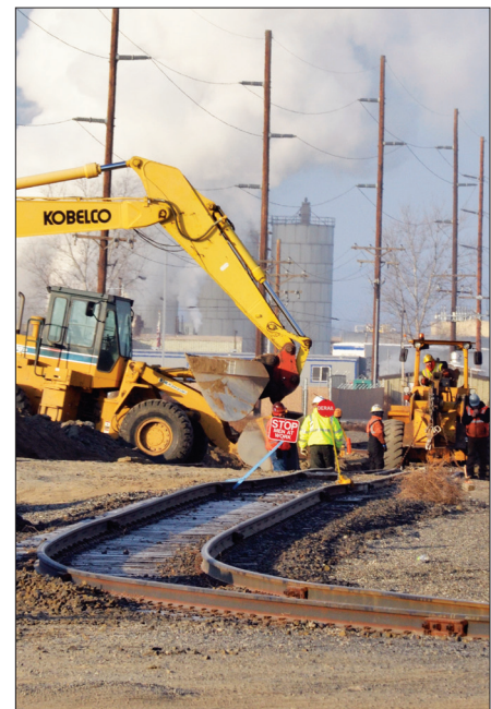
Track is installed at a new rail switch along Industrial Way at the Port of Morrow in early December 2013.
