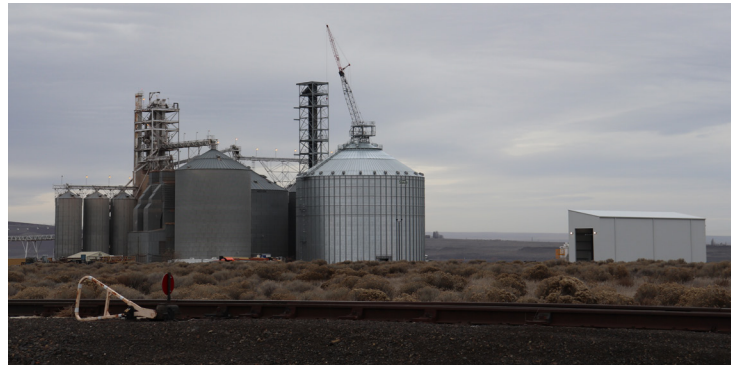
A new high-speed unloading facility is under construction at the grain terminal in Boardman.
