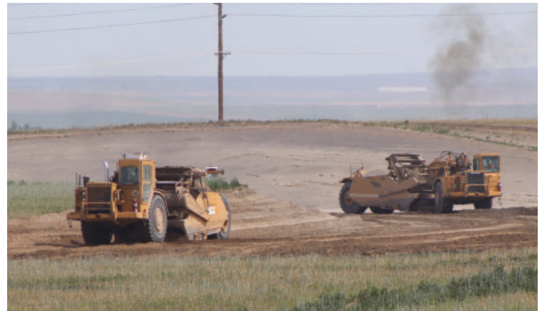
Earth movers prepare the new rail bed at the East Beach Industrial Park.
