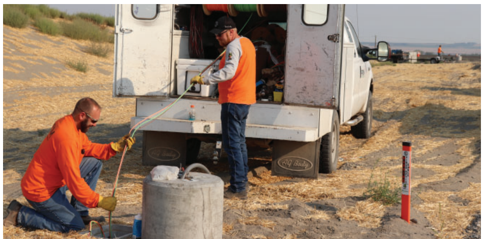
Purcell and Ezell feed wire through conduit for lighting along Gar Swanson while Falland pulls it through at the other end.
