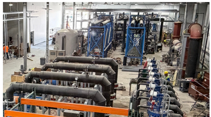
Advanced filtration systems will treat Columbia River water for use in the Port's industrial parks.
